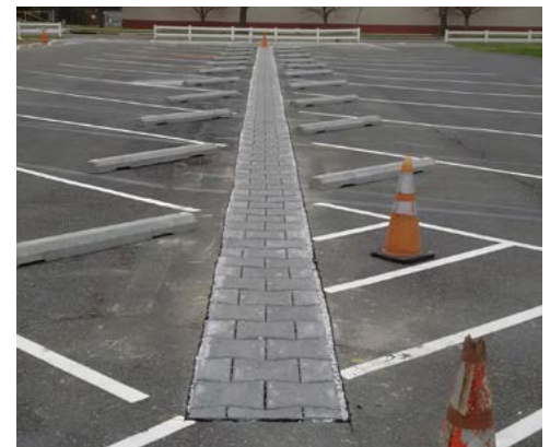
Innovative combination of an infiltration trench over permeable pavers at the Forestville New Redeemer Baptist Church.
